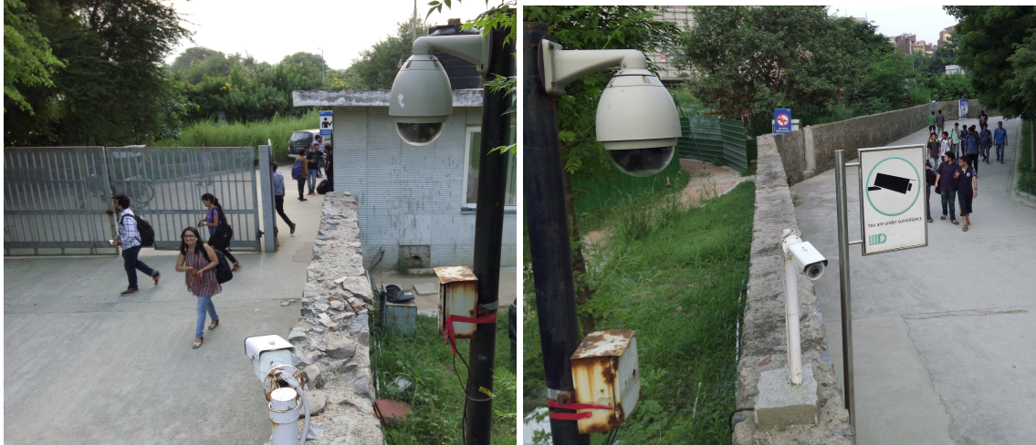
Figure 1-2: CCTV cameras can be installed for the purpose of surveillance. The images show CCTV cameras installed at entrance of a premise to keep record of the visitors.
